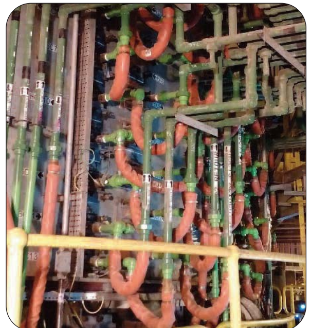
Typical water cooling sidewall hose assembly installation in a Pyrometallurgical nickel smelter with MSS SP 83 2006 3000 lbs socket weld unions
