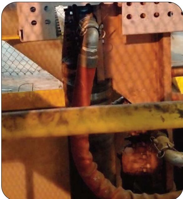
Thorburn's 48TSP-NC Furnace Door Hose Assembly with Cam-Lock Model 733 DBW Butt Weld Quick Coupling System installed at a Pyrometallurgical Nickel Smelter transferring dissolved chlorides
